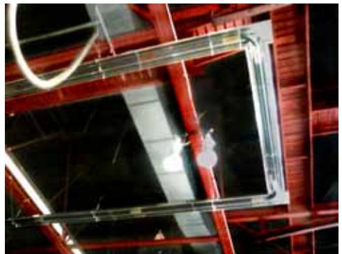
JMWA installed a Gas Fired Radiant Heat system, reducing the boiler system load and annual heating cost for large hangar.
