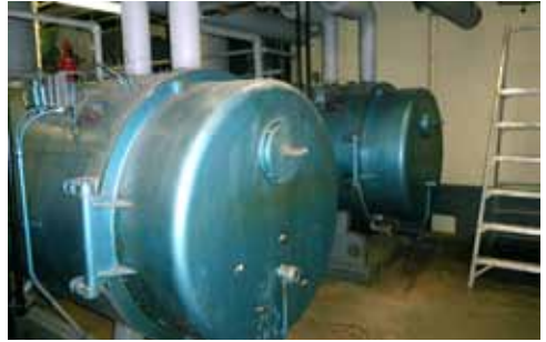
JMWA energy experts replace outdated equipment, such as this water boiler, with energy efficient models.
