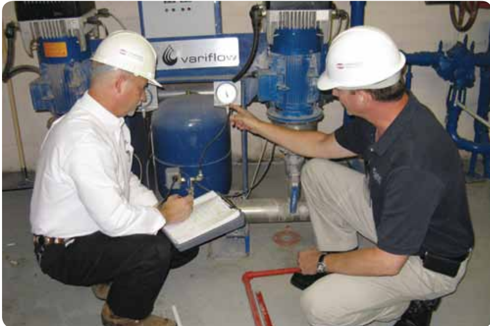
By assessing current equipment infrastructure, JMWA Asset Management Specialists can rapidly determine deficiencies and offer solutions.
